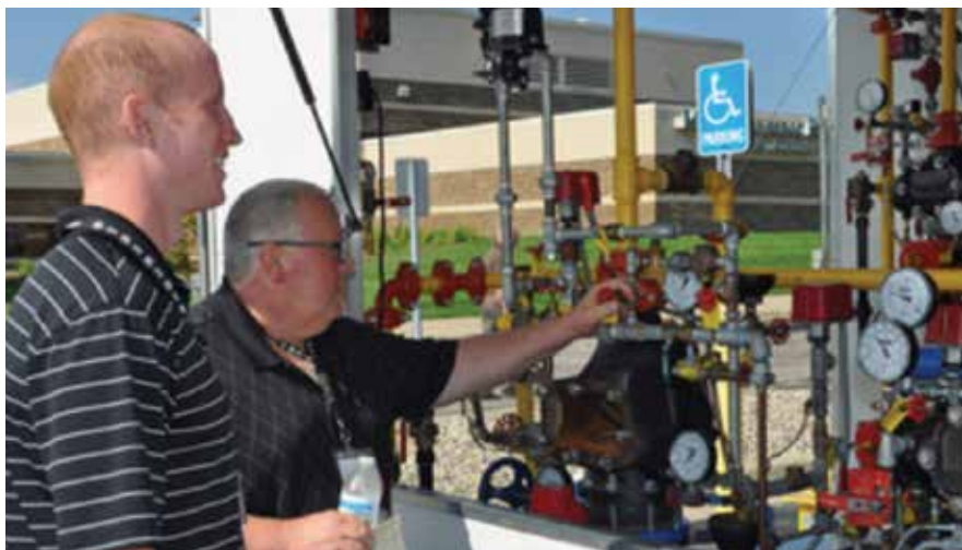
Photo caption: (From left) PCA member Patrick Birk (Birk Plumbing, Inc.) and Local 130 JAC Trustee, PCA Board Treasurer and PCA member Brian Kennedy (Gehrett Plumbing, Inc.) test out the UA mobile education trailers set up at the UA Industry Day in Ann Arbor, MI.
